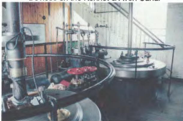
Part of the beam engines at Crofton. These engines pumped water into the Kennet and Avon Canal
