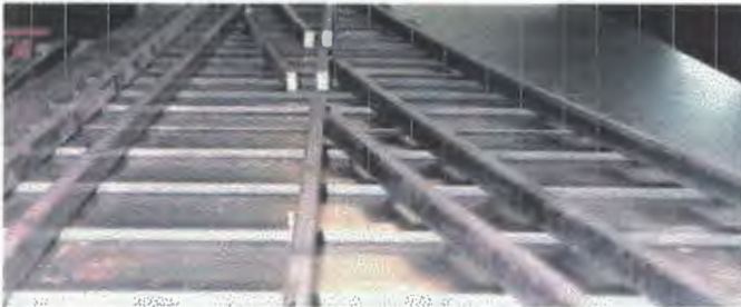
The first set of points is laid out on the points jig and will shortly be ready for welding.
